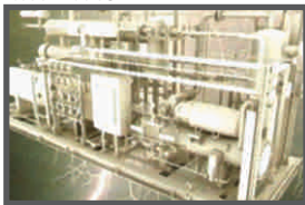
Cascade refrigeration plant NH3/CO2
