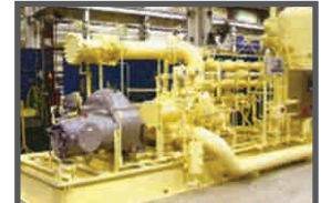
Screw compressor drive line
